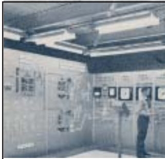
BANBURY CONTROL ROOM: Control panels for automatic banbury mixing equipment
